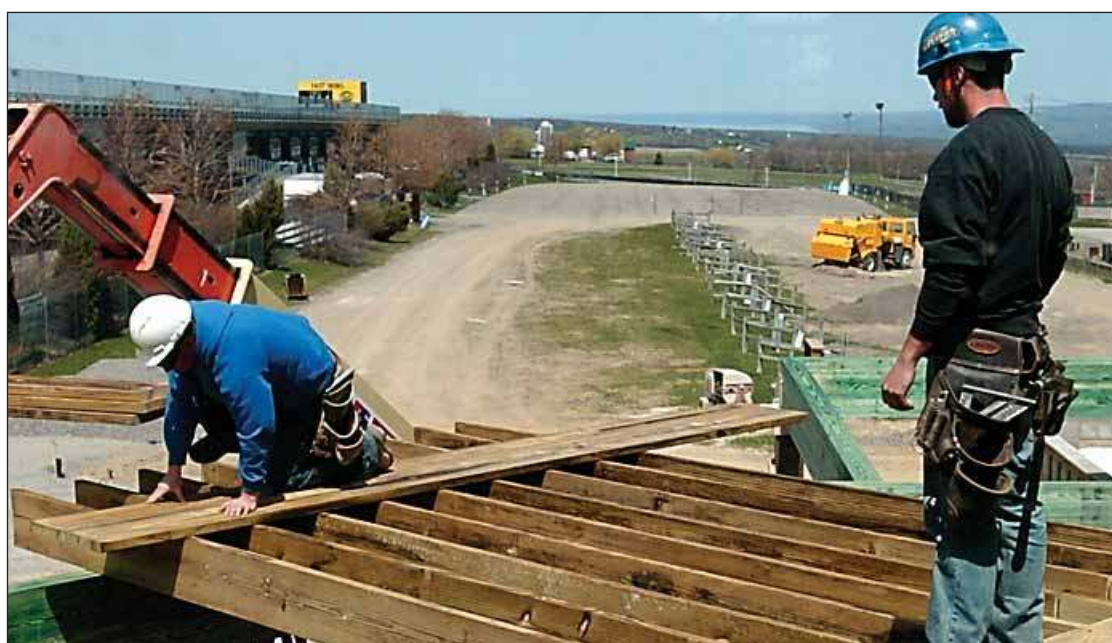
JASON COX | THE LEADER Construction crews work on installing a deck at the new WGI media center.
